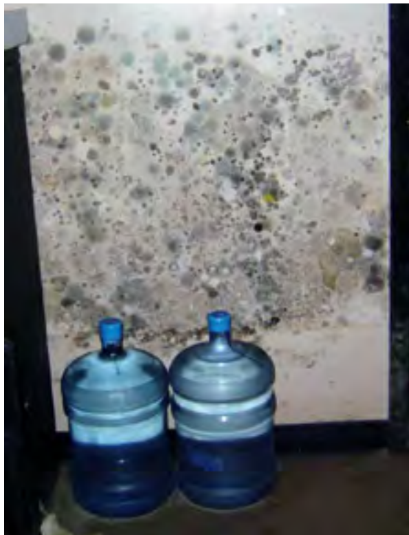
Mold growth on wall board.
