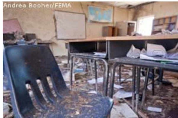
A School damaged by flooding after Hurricane Katrina.
