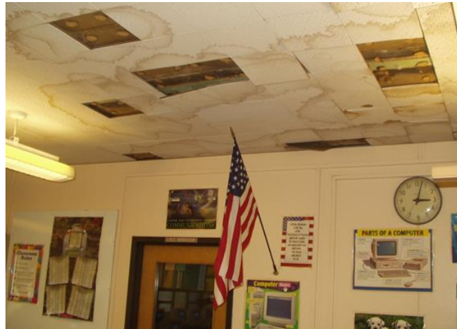
Water damaged, moldy ceiling tiles.
