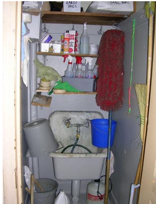
Inadequate, dirty janitorial closet.
